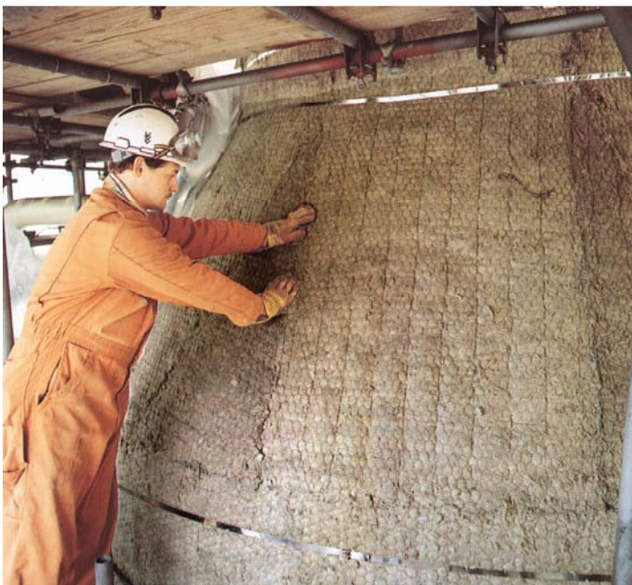
Mattress with Wire Mesh used as insulation for big vessels
